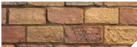
FIRE BRICK INTERIOR
